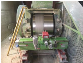
ZW Landquart, CH-Landquart Walzwerk: Rieter, 2012
